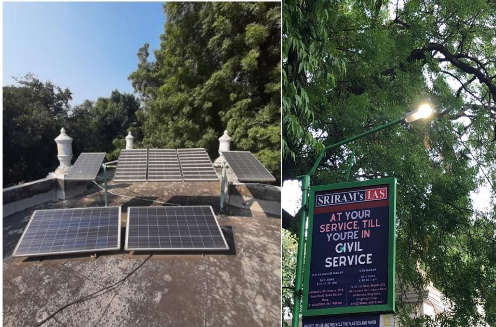
Solar panels and lighting in the campus
